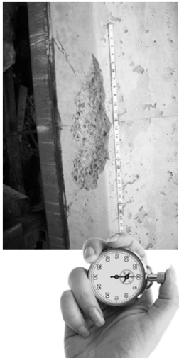
DAMAGE FOUND THAT APPEARS TO NEED REPAIR
