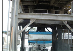
Batch plant discharge
