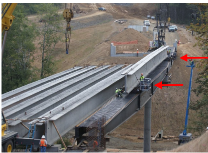
Motorized dollies move girder across the launching beams to the next span
