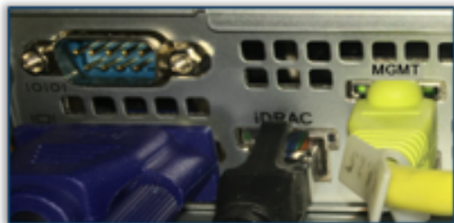
Figure 1 Management port location – Left Side
