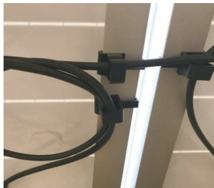
Wires routed outside and perpendicular to the frame member.
