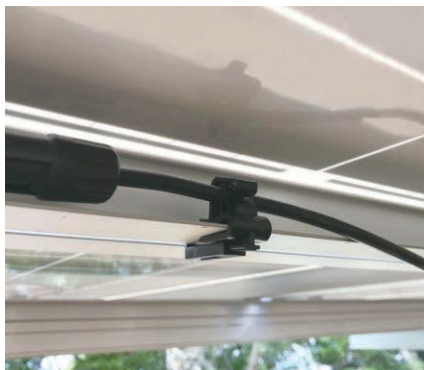
Wires routed inside and parallel to the frame member.
