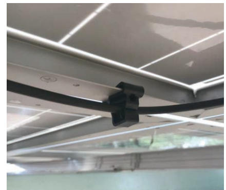
Wires routed outside and parallel to the frame member.
