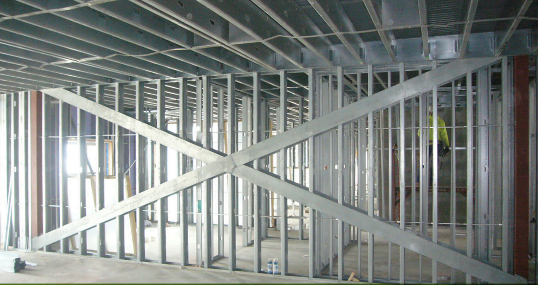
Metreau Apartments' lateral-resisting system includes X-braced CFS shear walls and pre-cast concrete stairs and elevator shafts.
