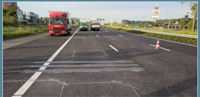
TACS Installation – Rotterdam, Netherlands
