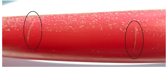
FIGURE 9. Exterior view of circumferential cracking resulting from a combination of mechanical stress from bending and chlorine-induced degradation
