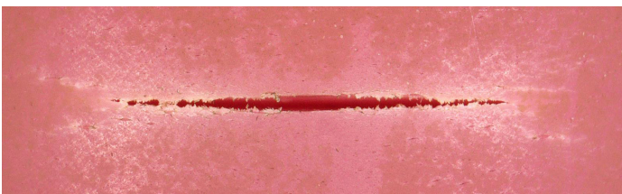
FIGURE 2. Through-wall crack, from interior (magnified)
