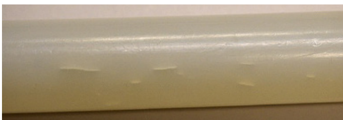
FIGURE 5. Stage 3 PEX failure from a system reported to experience intermittent water pressure spikes above 80psig in chlorinated water
