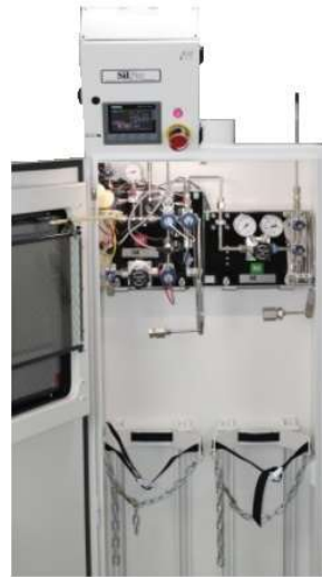
INSIDE CABINET PICTURE 1
