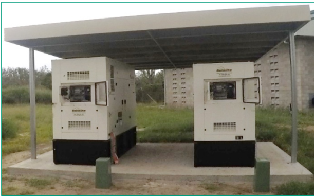
Figure 4: 450kW Standby Generation
