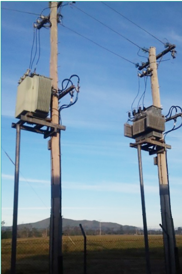
Figure 2: Existing 2 x 500kVA Pole Mount Transformers
