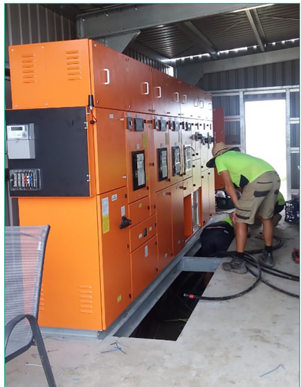
Figure 7: New Main Switchboard
