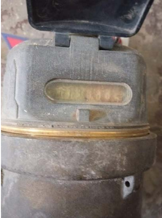
Old water meter – can't read water usage
