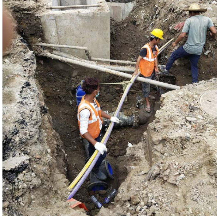
Lack of GIS/plans makes pipe repairs difficult
